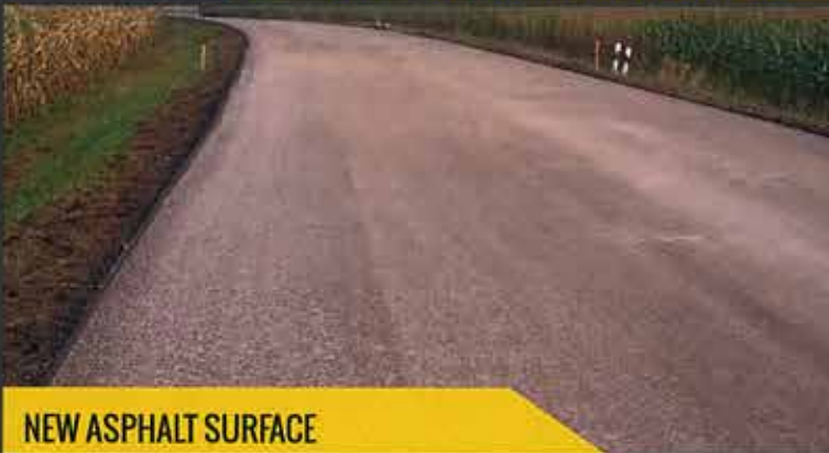
OLD ROAD WITH DAMAGED SURFACE
